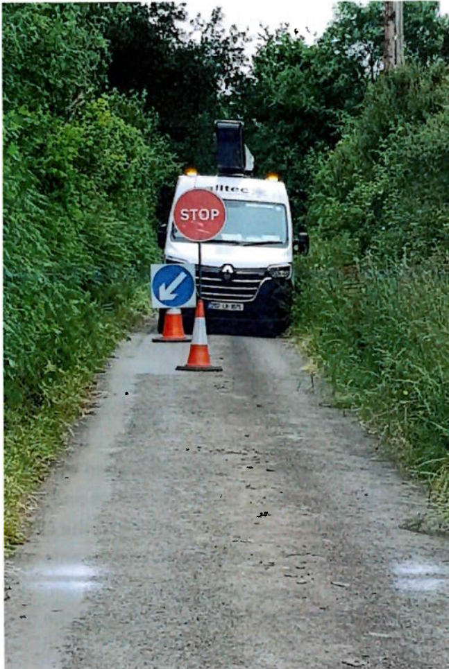
Our residential local road L70382, blocked during maintenance by a Telecoms company, 2022.
